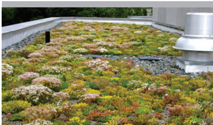
Fig. 4.23.2: Extensive sedum green roof
